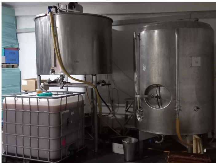
Another IBC nears full as the homogenising, left, and holding, right, tanks look on.
